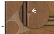
Knife Outs Tear outs along the edges of the door
